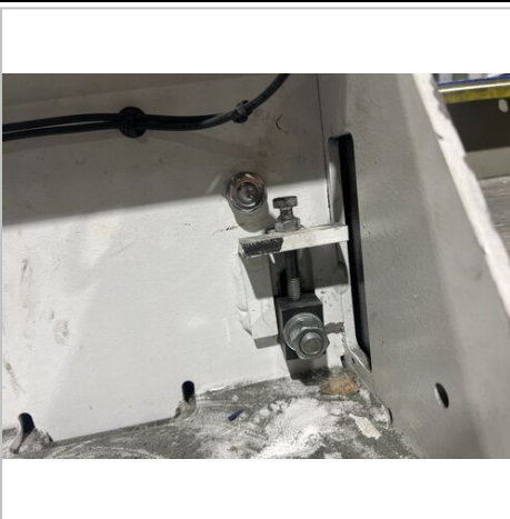
Chain tensioner set at max, requires new chains left hand side
